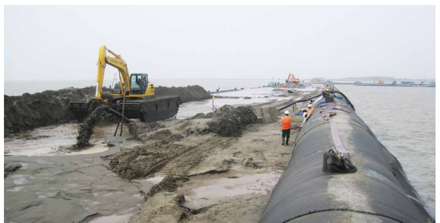
> The work platforms, together with the geotextile tubes, will eventually be embedded within a future land reclamation that will enlarge the Dinh Vu Development Area.
