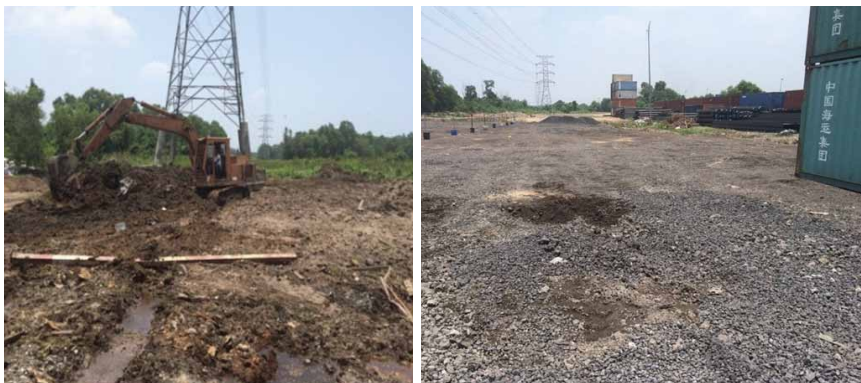
Figure 1: Rutting on container's load supporting platform
