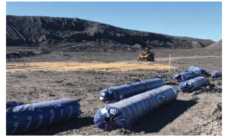
Reinforcement geotextiles delivered in custom roll lengths and installed using light Bobcat equipment. Each roll is individually marked to assist laydown works
