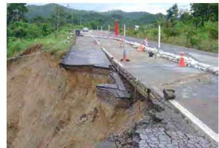
The erosive slip failure at Khun Tan, Lampon
