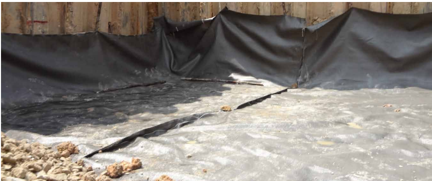
Installation of Mirafi® HP380a over the flat thin soil layer followed by aggregate backfilling.
